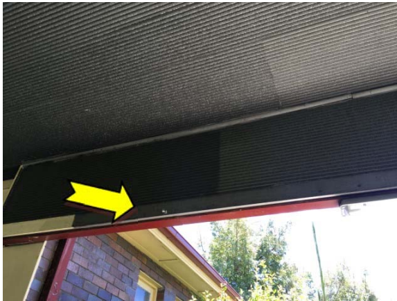
Photo 9. Exterior, upper height walls – suspected lead-containing upper green paint system.
