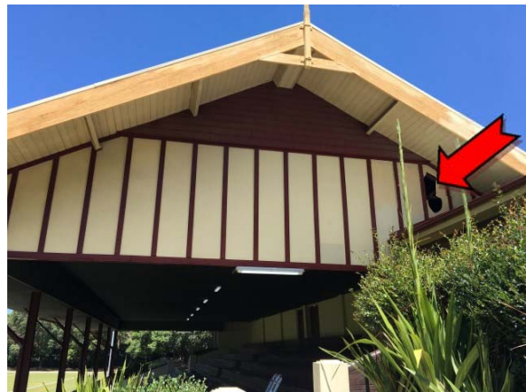
Photo 4. Exterior, north elevation, gable end – exposed suspected asbestos-containing fibre cement sheeting.
