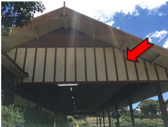
Photo 3. Exterior, south elevation, gable end – suspected asbestos-containing fibre cement sheeting.
