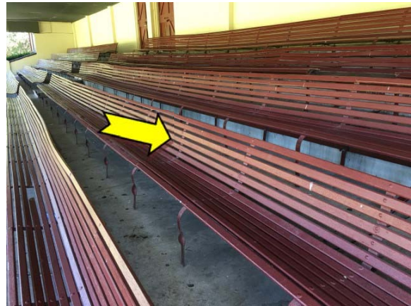
Photo 10. Exterior, grandstand, seats, doors and support columns – suspected lead-containing red upper paint system.
