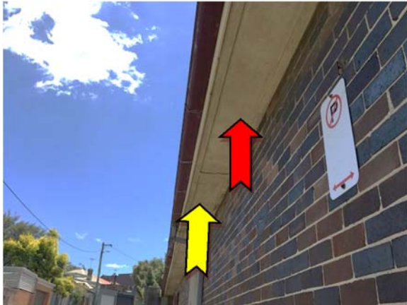
Photo 1. Exterior, west elevation, eaves – suspected asbestos-containing fibre cement sheeting and suspected lead-containing cream upper paint system.
