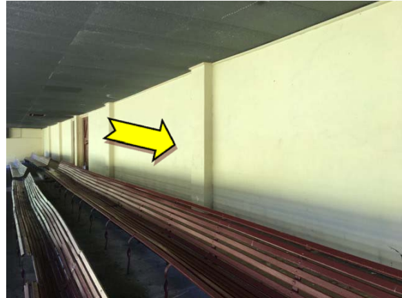
Photo 8. Exterior, throughout, walls – suspected lead-containing cream upper paint system.
