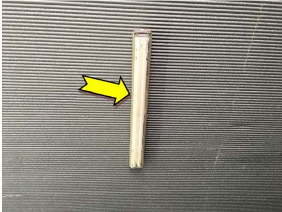
Photo 7. Exterior, throughout, double tube fluorescent light fitting – suspected PCB-containing capacitor.
