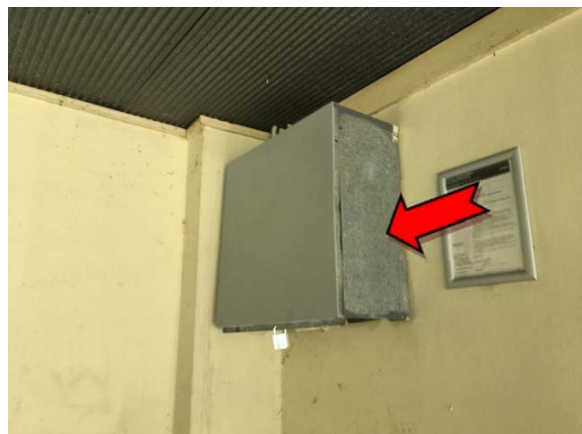
Photo 6. Exterior, north-west elevation, electrical board – suspected asbestos-containing bituminous backing board.
