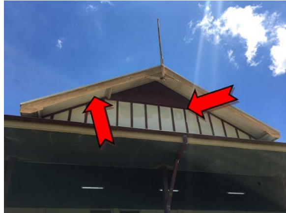
Photo 2. Exterior, east elevation, façade and eaves – suspected asbestos-containing fibre cement sheeting.
